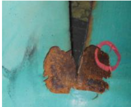
Figure 2. Crack arrest side O, with the paint peeled off around the plastic zone in front of the crack tip. This is typical of a classic Case I situation in Fracture Mechanics when the stress in front of the crack tip becomes lower than the yield strength, causing the crack to stop.
